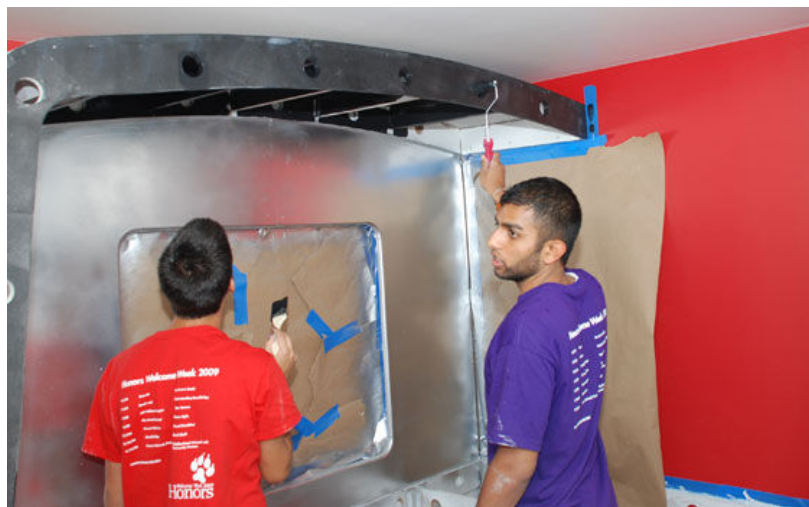
Students from Northeastern University paint as part of the renovations to Putnam Place on Glendale Street in Dorchester. The program houses young males between the ages of 15 and 22 who have either "aged out" of the Massachusetts foster care system or just grown exhausted of being shuttled back and forth from home to home as part of it. (Tony Irving photo)
